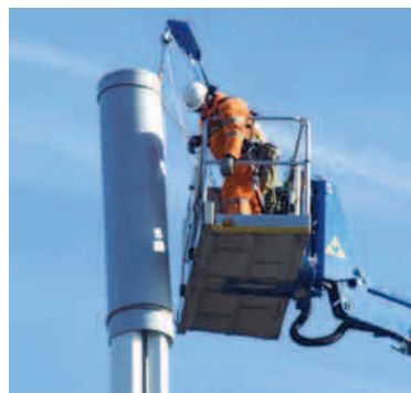
Nationwide Platforms' SkyTel antenna handling device was used beside a busy road
