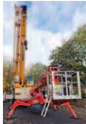
The Teupen Leo 36T spider platform was compact enough to be placed in front of the mobile crane
